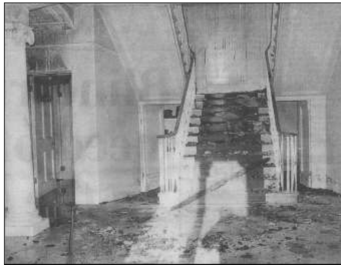
The Hall and Staircase after the fire.
