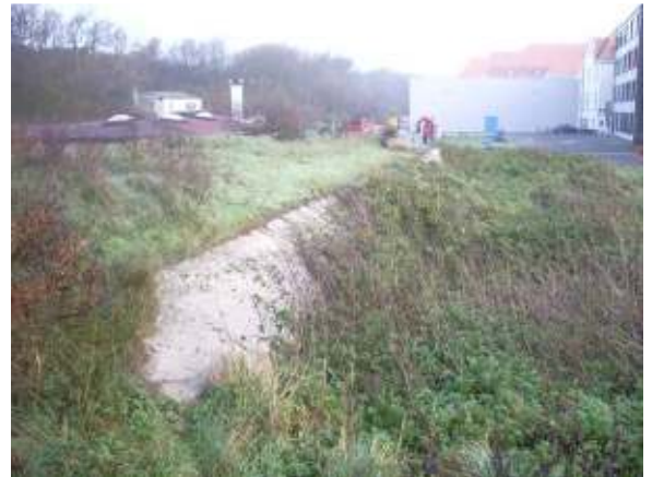
Today, only a small part of the roof is visible. We had to dig to reach inside
