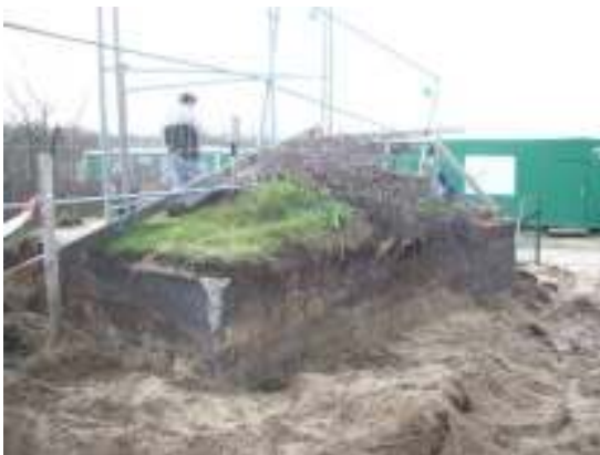
The VF Wasserbunker has quite small dimensions: 5,00 x 2,40 m with 0,50m thick walls
