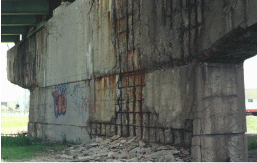
Figure 1 Corrosion damage in an elevated highway structure.
