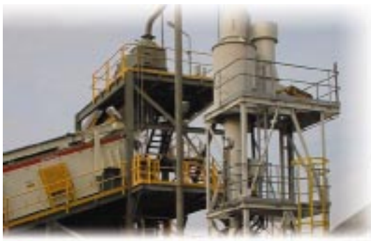
A DUST SCRUBBER WILL ASSIST TO CONTROL DUST.
