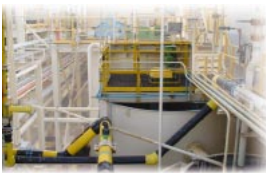
THE INCO CIRCUIT WILL DESTROY FREE AND WEAK ACID DISSOCIABLE CYANIDE.
