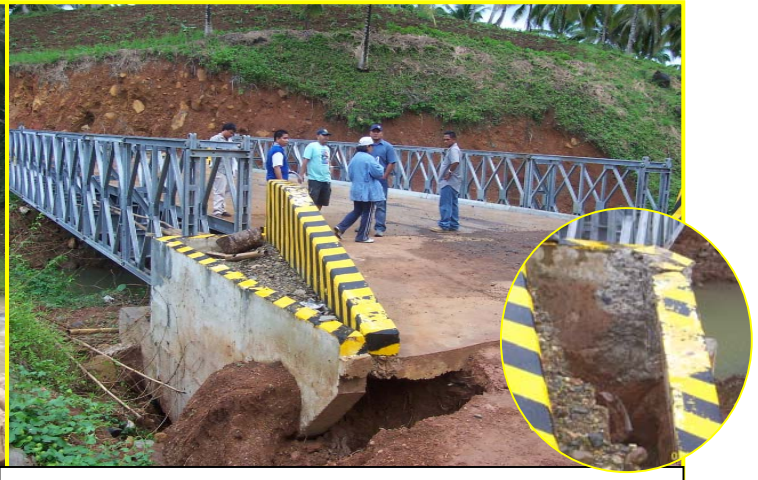
Payag Bridge in Malangas. The left portion of the approach eroded while the right wing wall (inset) of the bridge was damaged by flood due to non-removal of the detour bridge.
