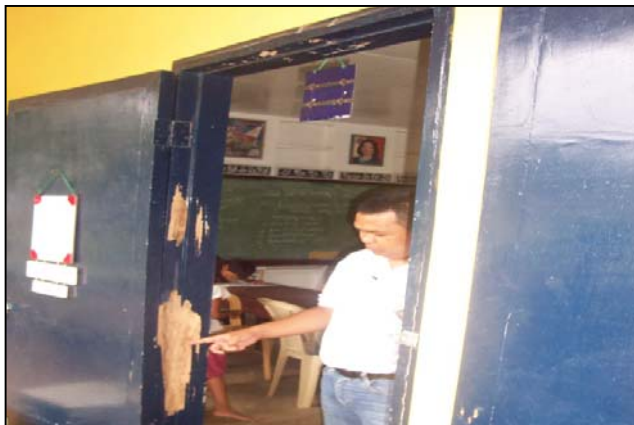
A teacher of Naga Elementary School pointing at the termites-infested door jamb of one of the school buildings under the TEEP project which was already completed.
