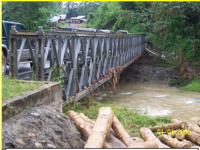
Bacalan Bridge in Naga. The elevation of the bridge is low, hence, if culverts at the downstream clog, water overflows
