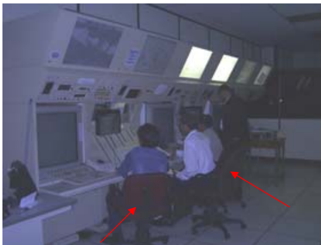
Figure 4. Chairs used by operators have the height 66-49 cm from the floor. Because the height of range of feet motion is only 63 cm, so that chairs cannot enter below the desk. Backrest cannot be used.
