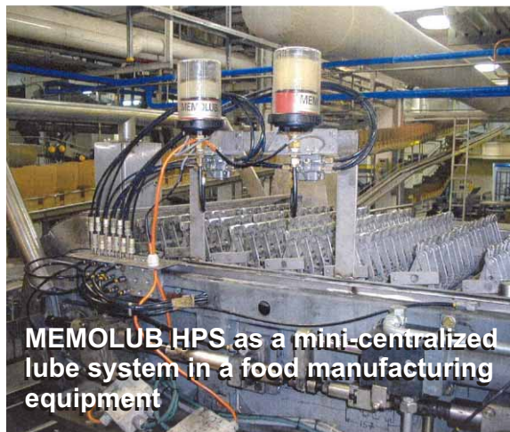
MEMOLUB HPS installed in a more accessible position
