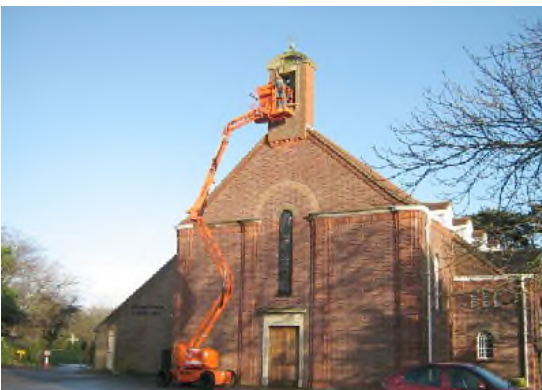
Up there fitting the new cable to the clapper
