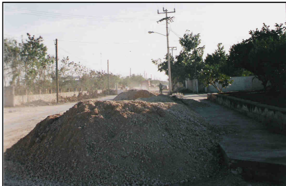
A view of the new highway construction going on in front of the school. The wall (recently knocked down) on the left, fronts the new neighborhood.
