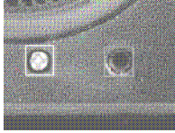
One screw missing
