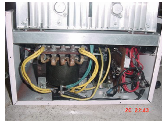
Tampak samping Trafo & Diode Bridge
