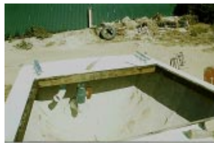
There is a ply deck on the opening with a smaller hatch in it.
