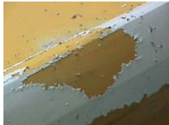
Figure 3.48. Only slight blistering of the coating occurs after application of the solvent.
