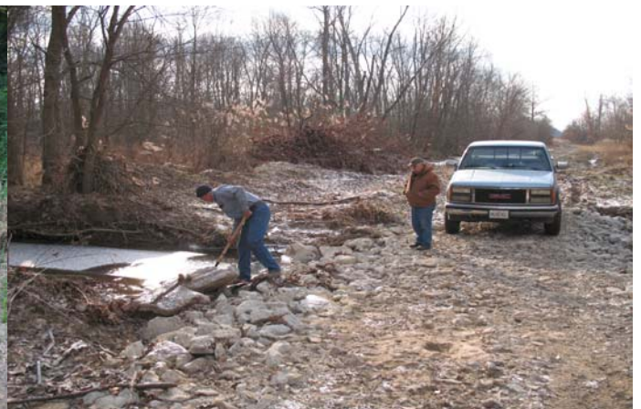
In the picture below, volunteers work to maintain the completed low water crossing.
