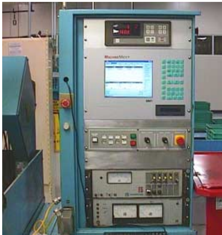
MachineMate CNC and Machine Tool Builders Panel retrofit into old cabinet
