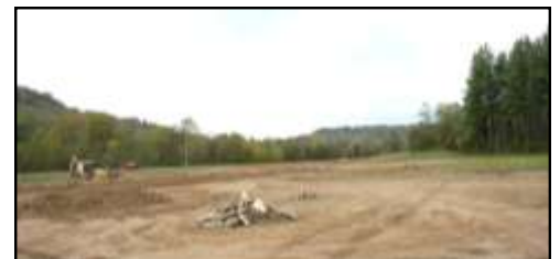
Shown here during construction is a view of one of the "islands" which may attract water fowl and will also serve as habitat for aquatic life.
