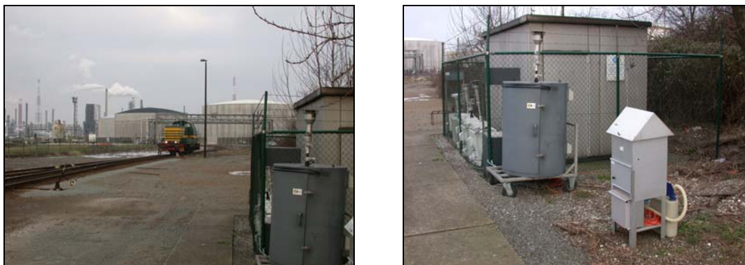
Figure 7: Typical set-up at Antwerpen-Petroleumkaai
