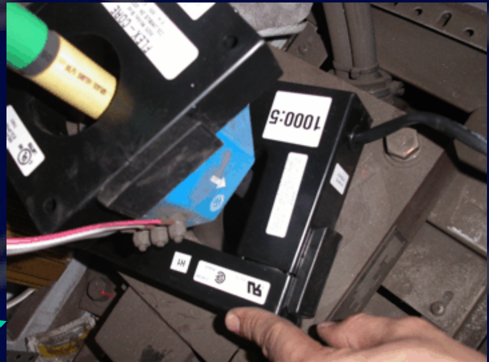
Hall-Effect Current Transducers Clamped on Return Conductor
