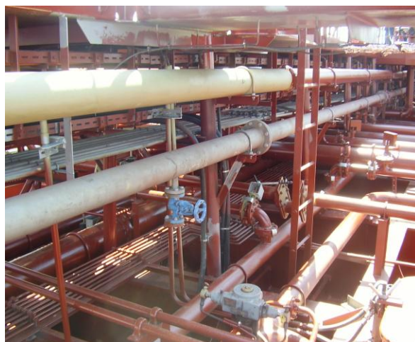
Figure 7: Cargo pipes on the main deck
