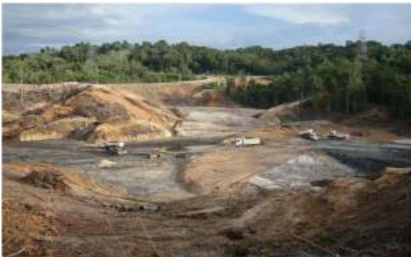
Date : 25-Sep-10 Description : Zone A P10 Earthworks is progressing at Sub-zone A2.
