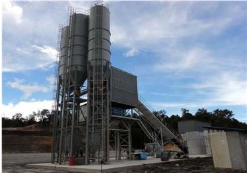
Date : 25-Sep-10 Description : Concrete Batching Plant Area P12 View of the completed.
