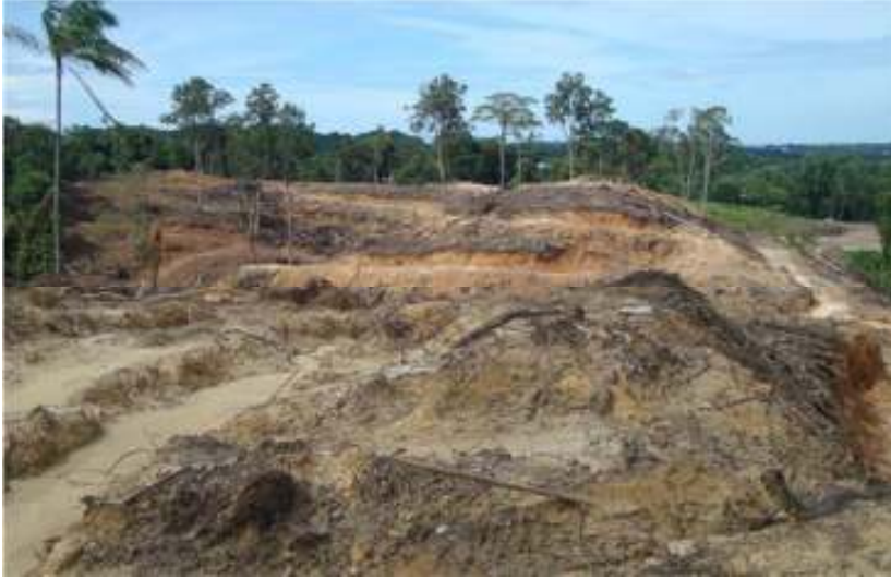
Date : 25-Sep-10 Description : Zone D P3 Site clearing is progressing at Sub-zone D1.
