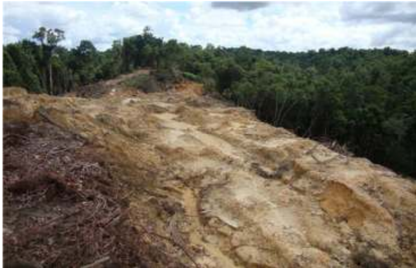
Date : 25-Sep-10 Description : Zone D P4 Site clearing is progressing at Sub-zone D1.
