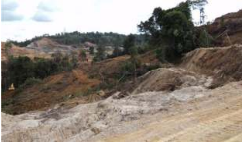
Date : 25-Sep-10 Description : Zone A P13 Site clearing is progressing at Sub-zone A1.
