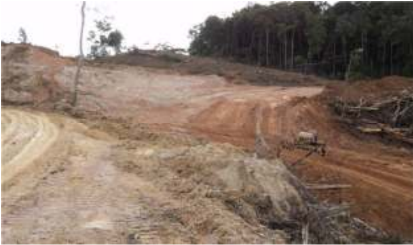
Date : 25-Sep-10 Description : Zone A P14 Preparation of access road at Sub-zone A1.
