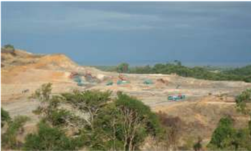
Date : 25-Sep-10 Description : Zone B P8 Earthworks is progressing at Sub-zone B1.
