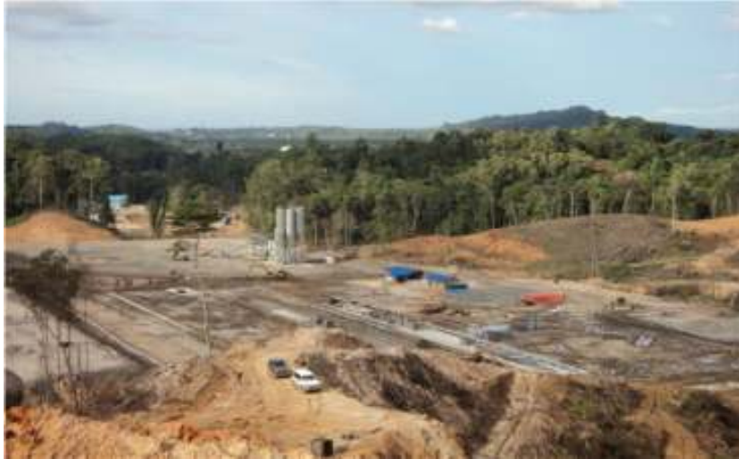
Date : 25-Sep-10 Description : Concrete Batching Plant and Casting Yard Area P11 Overall view.
