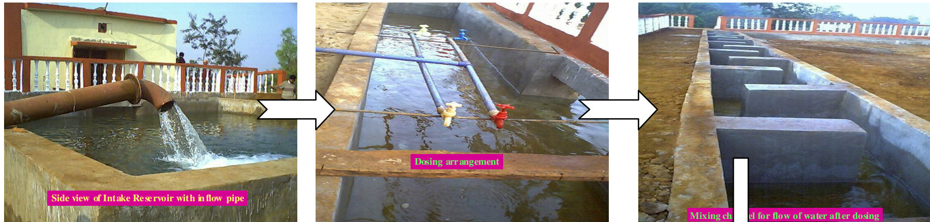
Fig. 5 : Effluent Treatment Plant at Sukinda Mines (Chromite)
