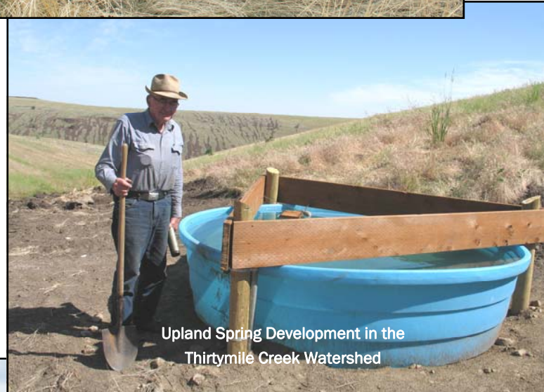
Livestock and Wildlife Watering Project with Well
