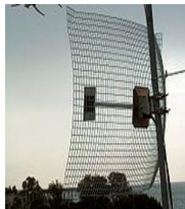
A roof mounted Wi-Fi antenna
