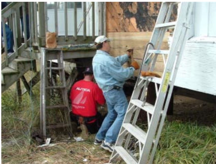
Matt Crocker and Charlie Pencinger, VFC, making carpentry repairs at the boathouse.
