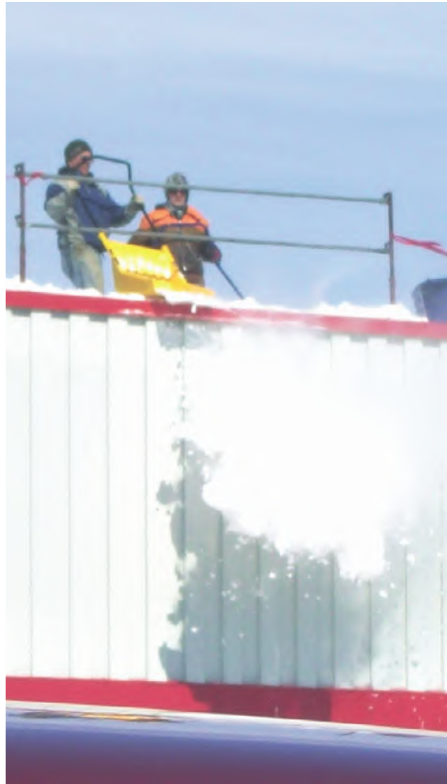
Above, left: Micheal Chatelois took these pictures of workers shovelling the snow off the roof of Zellers store last week. Right: Review freelance photographer Sylvain Lauwers took this photograph showing his daughter, Rachelle shovelling off the roof of her playhouse recently.
