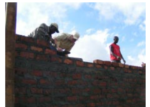
Above and below: David helping a masonry team build the second phase of buildings for a tuition-free Christian school.
