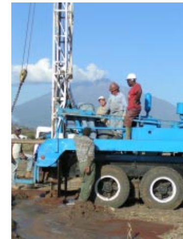
David with the well team on the drilling rig in the Kisongo village.
