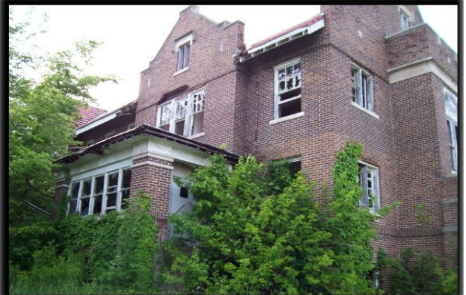
Bottom: The building will soon be swallowed up by weeds.
