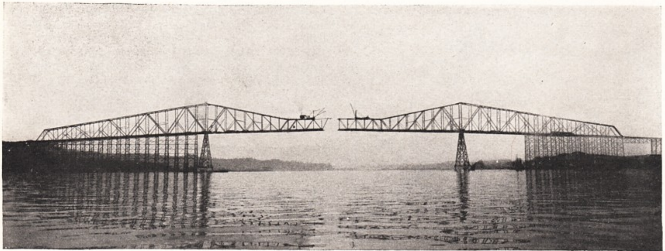
FIG. 1—LAST MOVE OF THE TRAVELERS ERECTING THE 1,200-FT. CANTILEVER SPAN OVER THE COLUMBIA RIVER AT LONGVIEW, WASH.
