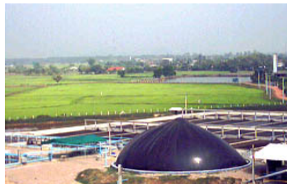
Fig 8: Bunmi Farm's biogas plant [2]
