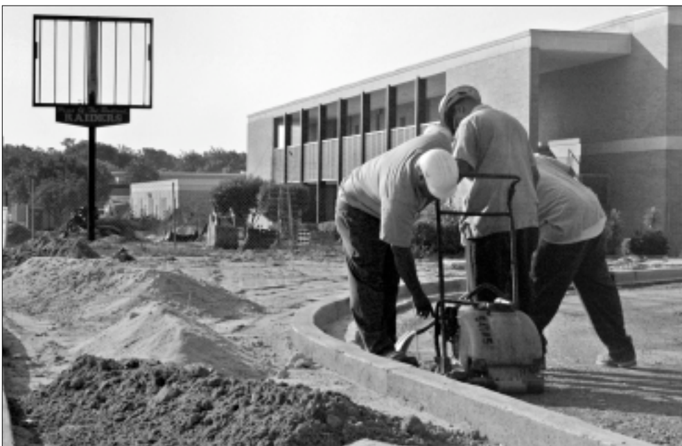
Sanders Middle will be relocated to the former Keenan High campus on Pine Belt Road. Additions to the facility will include new classrooms, practice gyms, two science labs and a performing arts area. This project is slated for completion in December 2009.
