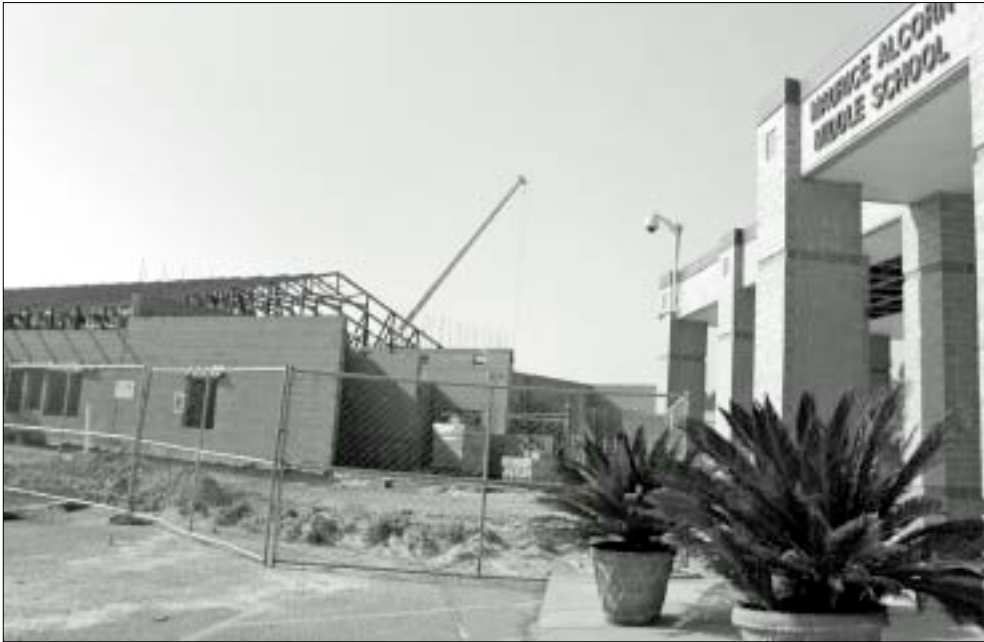
New classroom wings, an auditorium and a performing arts wing are being added to Alcorn Middle School. The project is scheduled for completion in December 2009.
