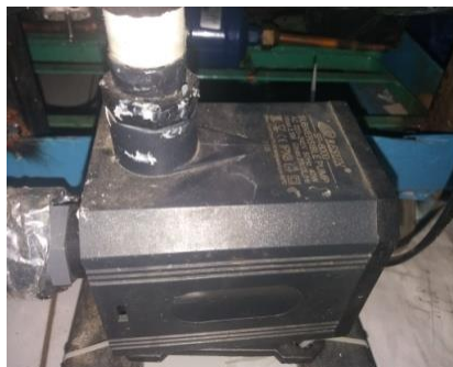
Figure 10. Cold Water Pump
