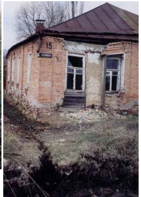
A house that has been damaged by the slow flooding
