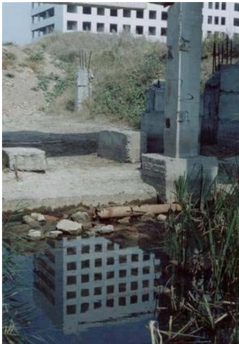
Flooded area in building site since the site work was stopped in early 1990s
