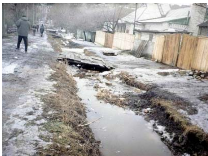
Snow water floods a street drain in one-family houses block
