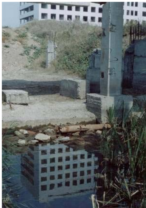
Flooded area in building site since the site work was stopped in early 1990s
